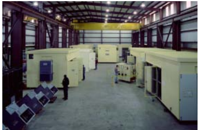
Manufacturing Plant Assembly Bay with Integrated Power and Control Buildings
