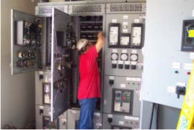
Control Cable Termination
