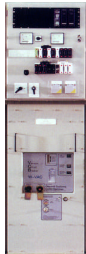
High Voltage Switchgear
