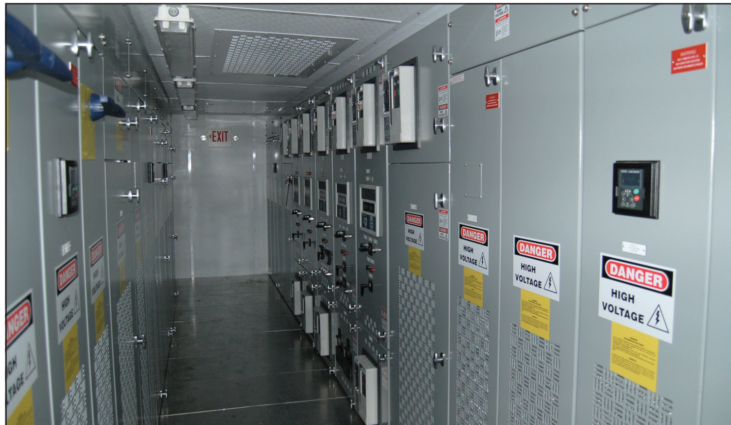
AC Drive System installed in Powerhouse including 6-VFD Drives
