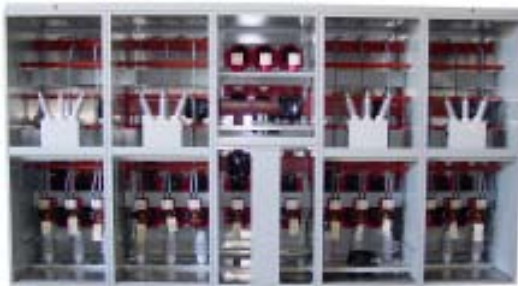
15KV Switchgear, Rear View
