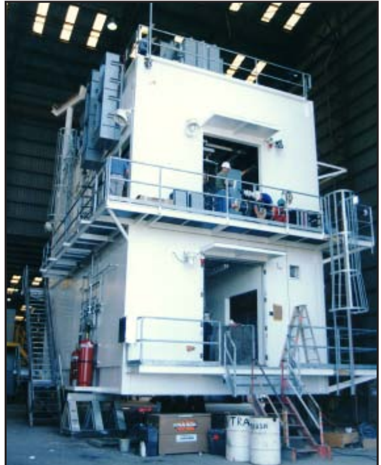
Offshore Module Including Medium and Low Voltage Switchgear, Bus Duct and Motor Control Center
