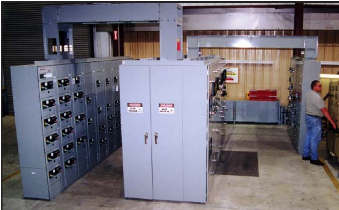
Switchgear, Motor Control and Bus Duct in Factory Test Bay
