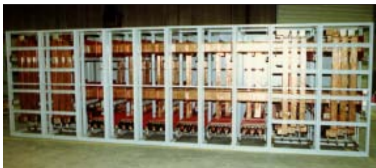
Custom Switchgear with 12,000 Amp Bus and 130KA Bracing
