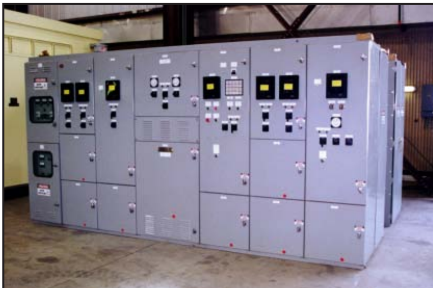
480VAC Generator Control and Distribution Switchgear
