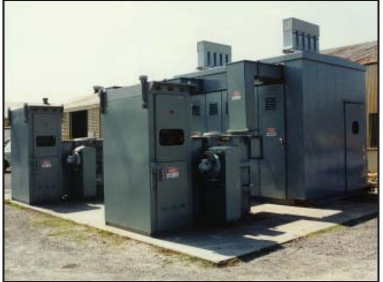
15KV - 480VAC Substation with 15KV Metal Enclosed Switchgear, Transformer, Bus Duct, Integrated Power and Control Building with 480VAC Switchgear and Motor Control Center
