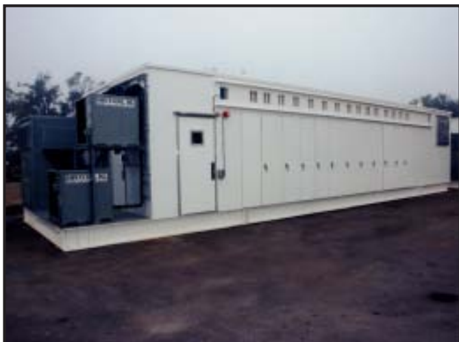
Packaged Substation Including 600VAC Switchgear, SCR Drives, Transformer and Motor Control Center
