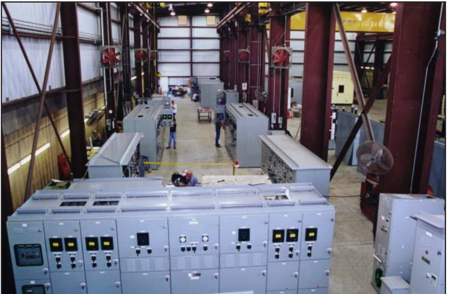
Manufacturing Plant Assembly Bay
