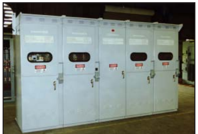
15KV Metal Enclosed Switchgear
