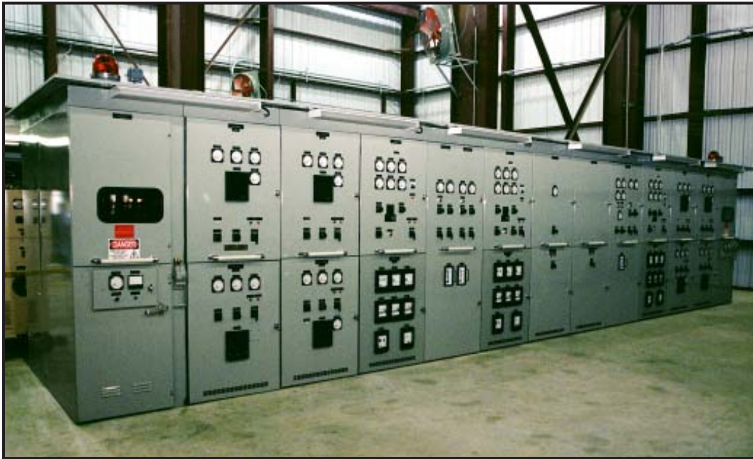
6.6KV Metal Clad Generator Control and Distribution Switchgear
