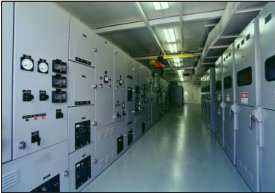
Integrated Power and Control Building Including 15KV metal enclosed switchgear, 5KV metal clad switchgear, 480VAC switchgear and motor control centers, marshalling cabinets, DC system and Class 1 Div II purging system
