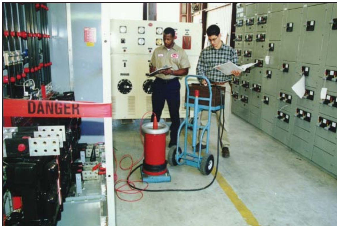
Switchgear Testing & Quality Assurance
